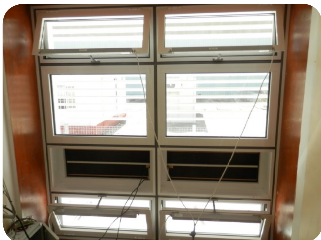
Façade prototype system with the motors installed and connected under monitoring
